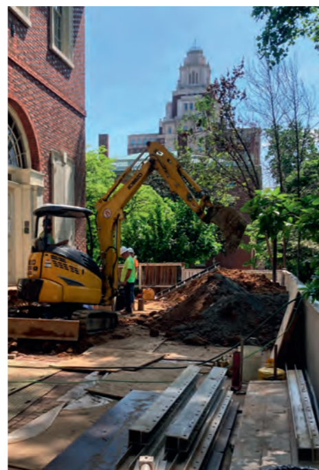
Perimeter excavation begins! An eight-foot-deep trench is being dug around the entire building to expose the original rubble foundation for waterproofing
