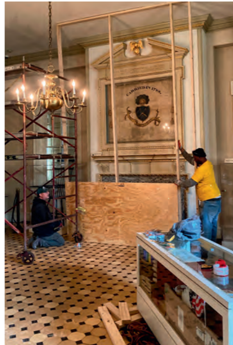
Workers install plywood covers to protect one of our historic banners, made in 1788 to celebrate the ratification of the US constitution
