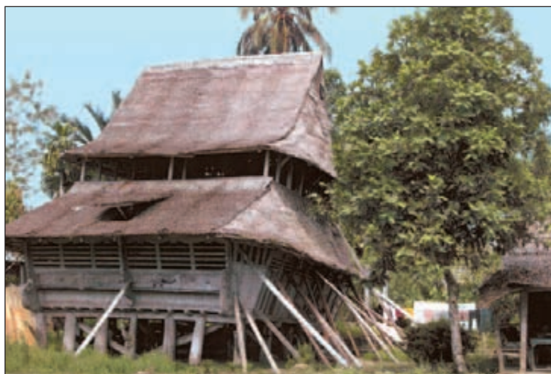
Wood house in Nias after the earthquake struck
