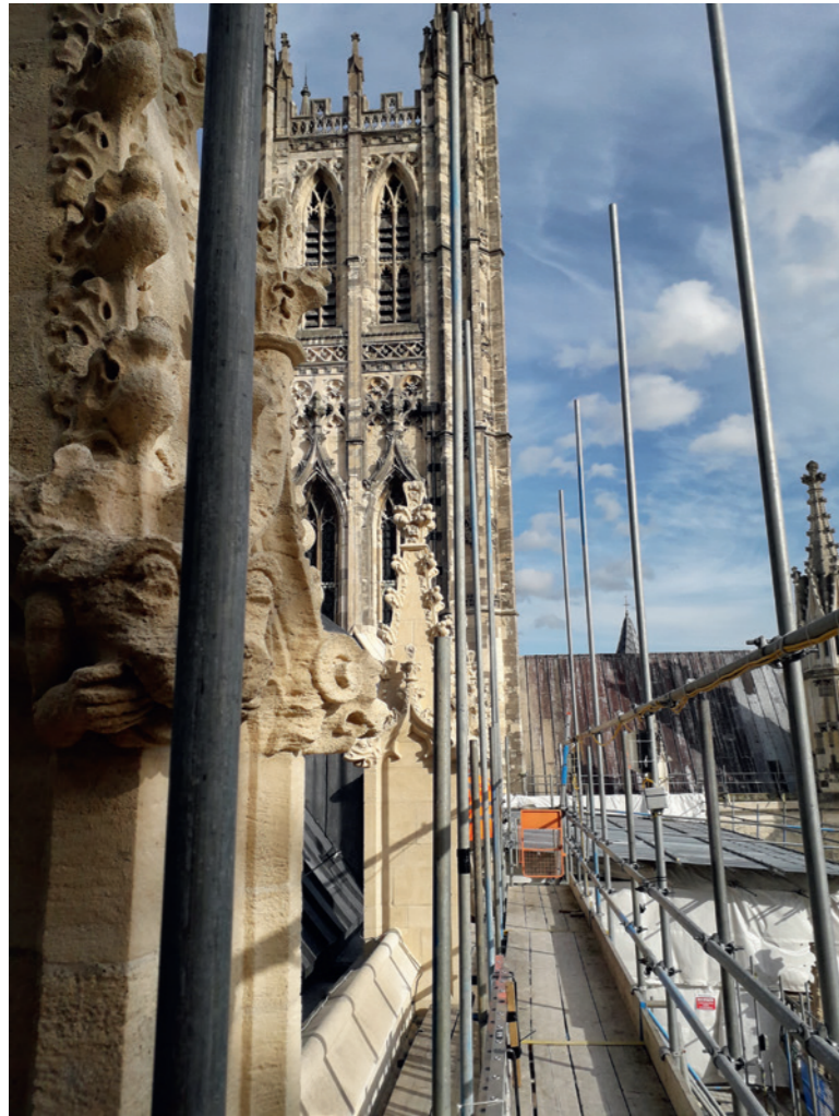
A close-up view of the ongoing work to the roof and towers
