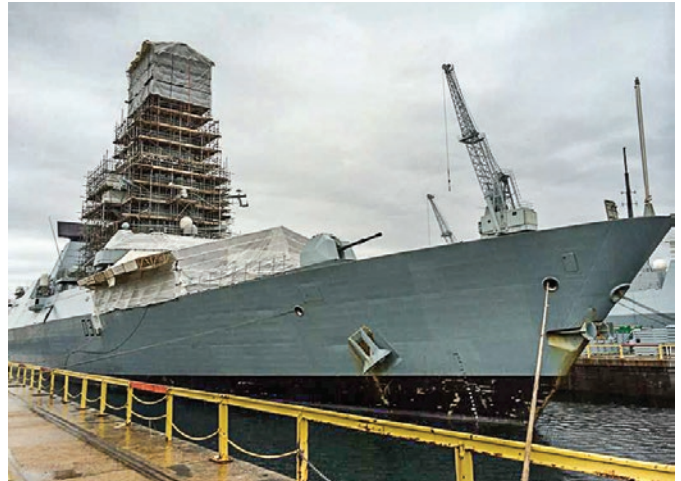
The foremast of HMS DARING shrouded in scaffolding as part of the lightning rod replacement and many communications upgrade work. The fo'c's'le aft of the medium calibre gun tented to undertake the Harpoon surface-to-surface missile system installation.
